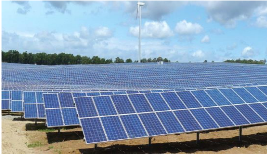
Location: Benevento, Campania, Italy Project Type: Ground Mounted Project Scale : 3 MWp
