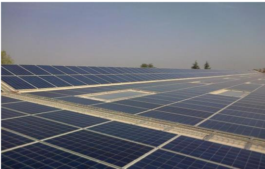
Location: Campania, Italy Location Type: Roof Top Project Scale: 1,3 MWp
