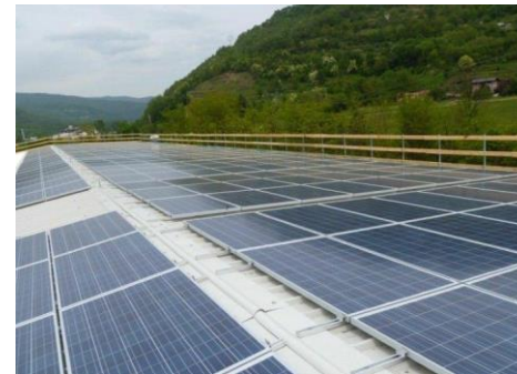
Location: Campania, Italy Project Type: Roof Top Project Scale: 1.8 MWp
